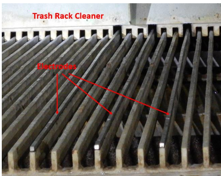
Figure 4. Fixation of electrodes for functional tests at the water intake of a nuclear power plant.
