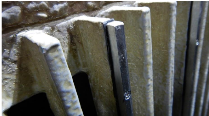
Fig. 6. Retrofitting of electrodes at the upstream side of the bars of an existing screen
